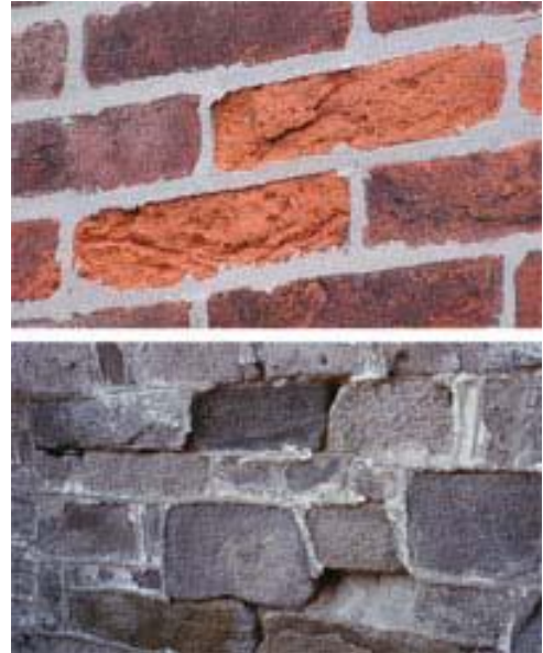
The results of too-hard mortar can be spalling of soft, pre-1860s brick (top) and some soft stones such as rubble fieldstones (bottom).
